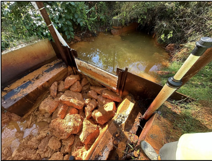
The newly installed weir at Crabtree was raised during a mine pool flow experiment and for the first time the discharge ran dry (for a few days anyway!)
