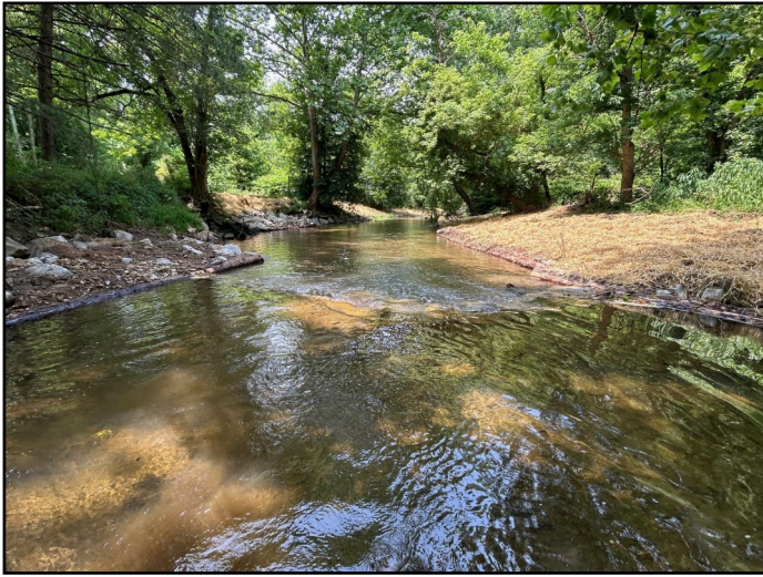
This log framed stone deflector and cross vane with rock throat was constructed on Mill Creek just above the confluence with the Loyalhanna.
