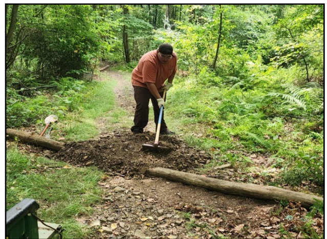
YCC Summer Intern Nolan Brahosky works to repair a wet section of trail using shale and logs.
